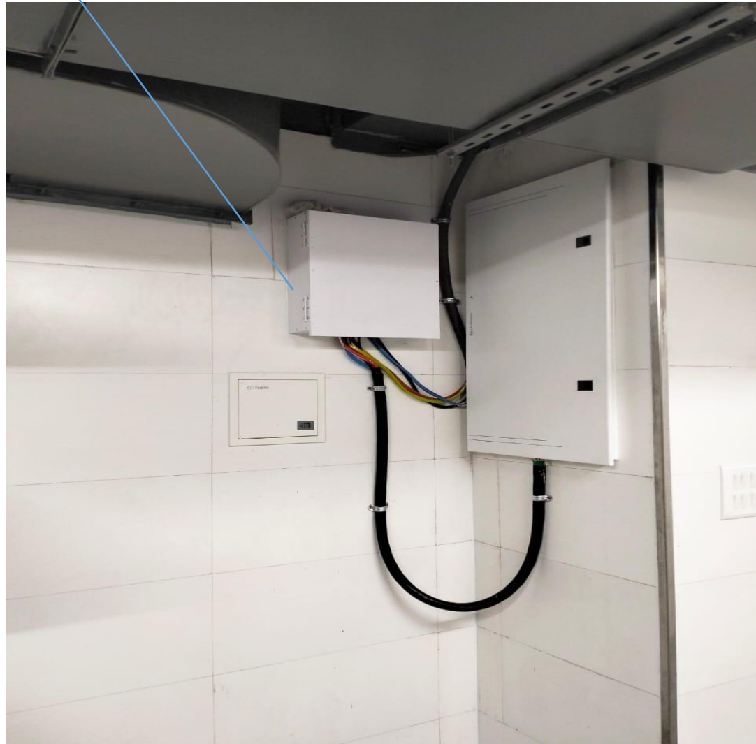
Line- 6 -Wooden Meter Box
