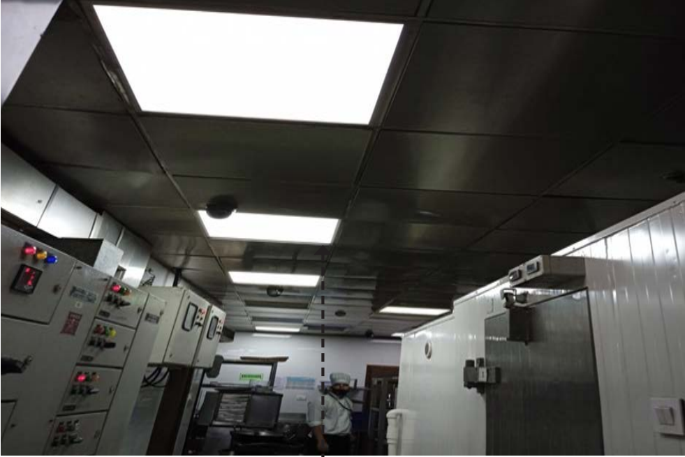
The ceiling in the picture needs to be completely changed with lights.
