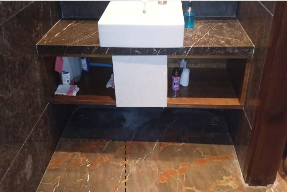
Washroom marble needs polishing.
