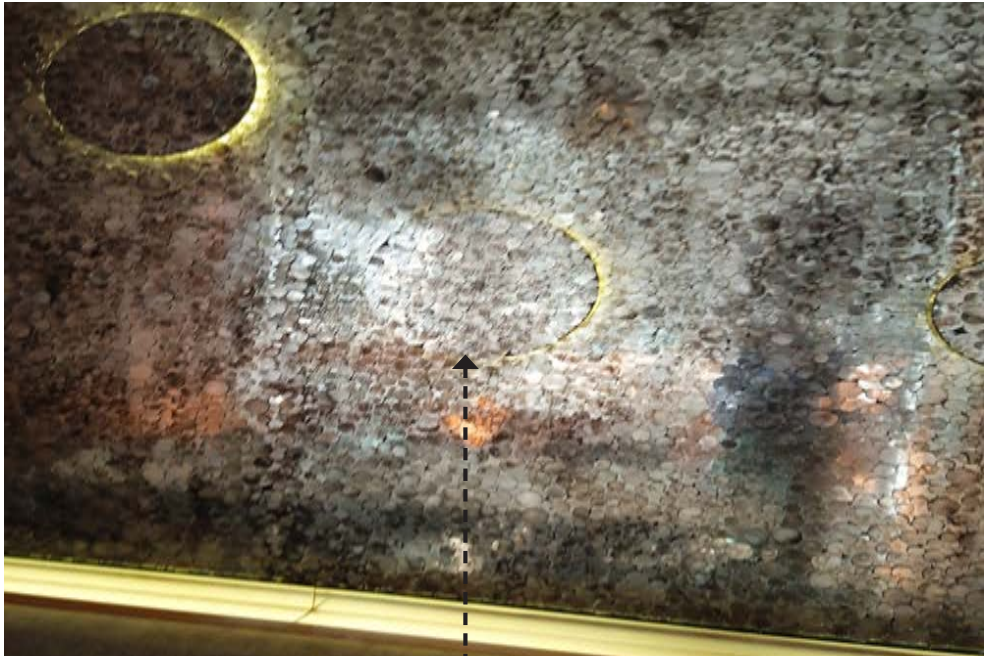
All 3 PDR rooms, need Tikli Work.
