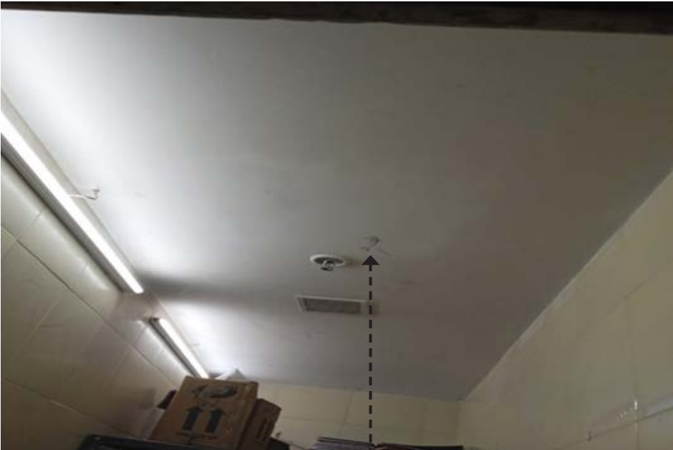
All Ceilings need repainting.
