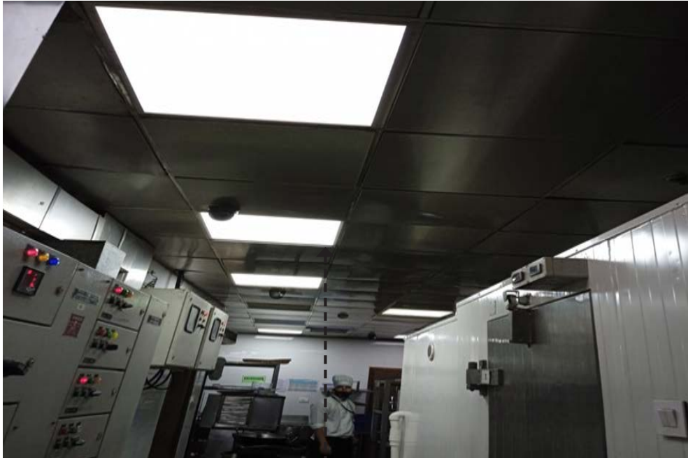
The ceiling in the picture needs to be completely changed with lights.
