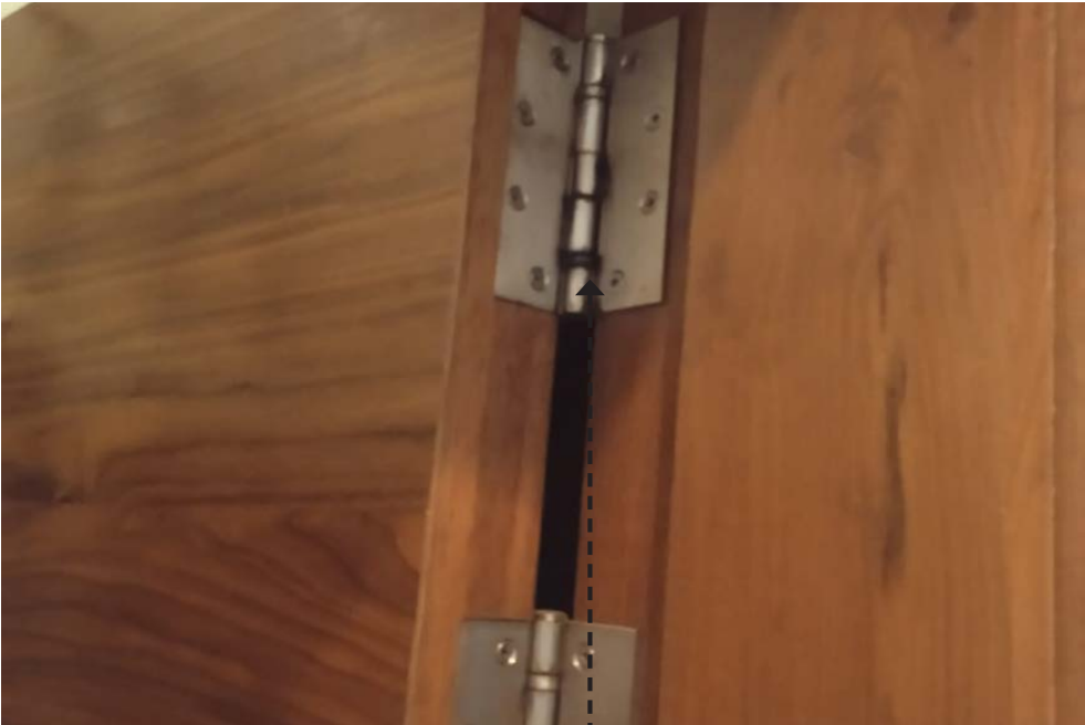
All Doors Hinges and Handles need to be changed.
