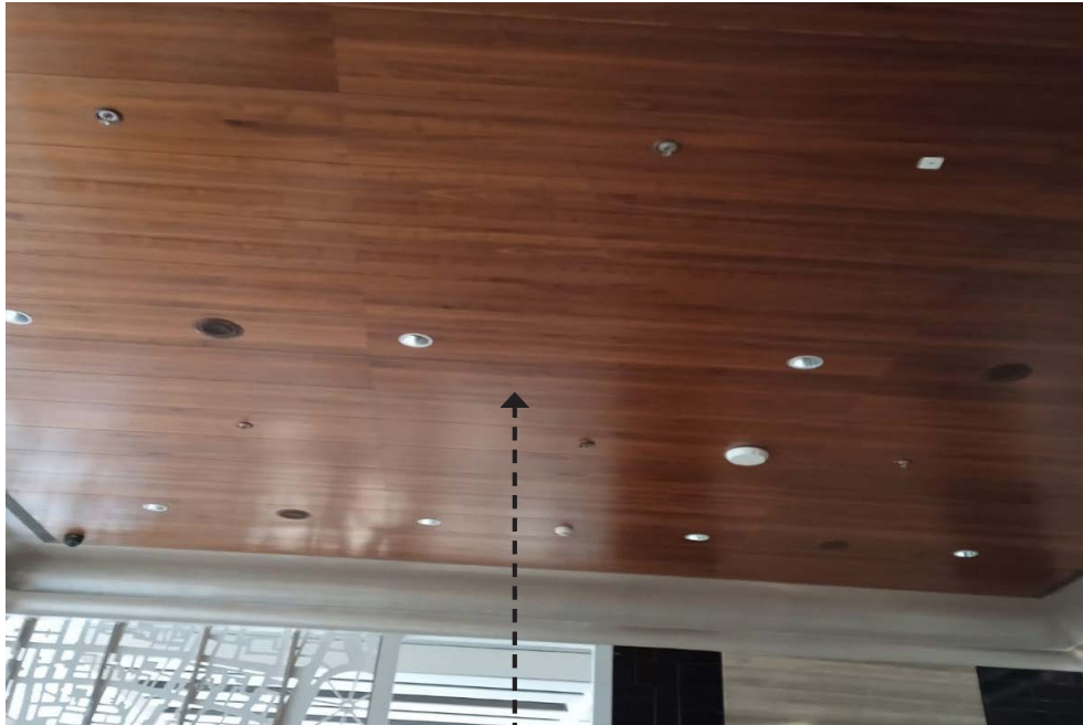
All veneer need to be replaced and then polished. The lights here need to be replaced with news ones as they have becomes dull.
