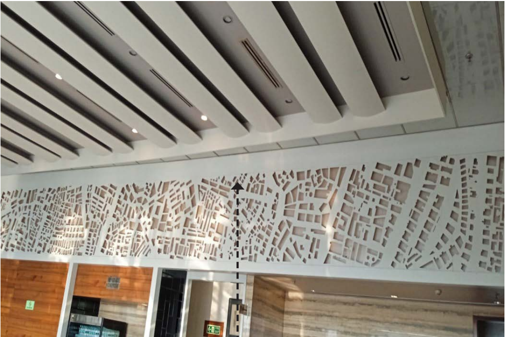
The ceiling needs painting.
