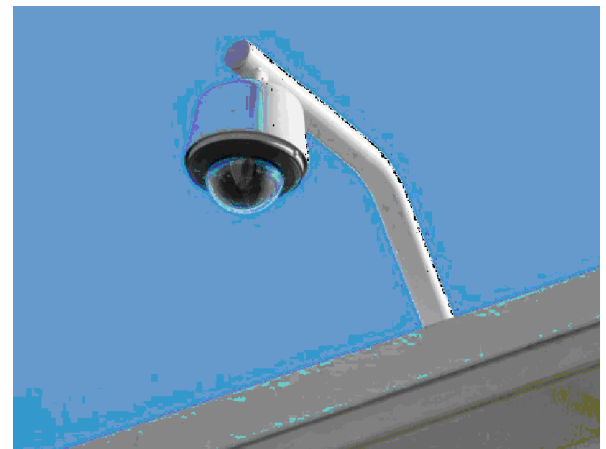
CCTV HANG ON WALL WITH MS SUPPORT
